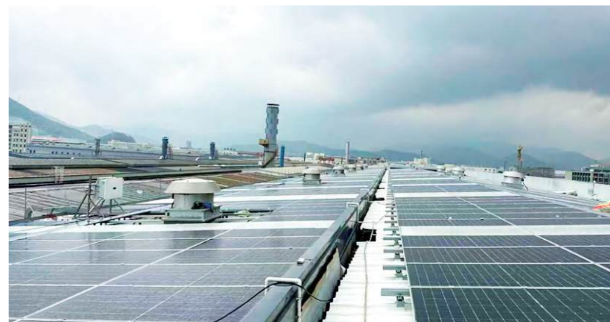
All six container factories under Shanghai Universal are equipped with PV power stations.
